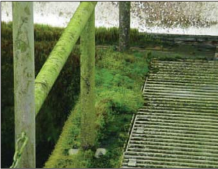
Algae slime on cement and metal
