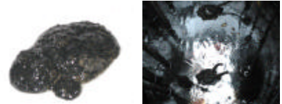
Lift station with oil and solids
