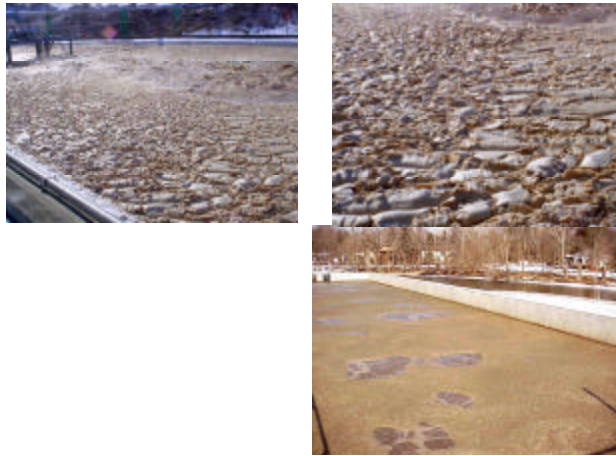
Here are some plants with tons of Nocardia foaming due to grease and high solids handling in the clarifier.
