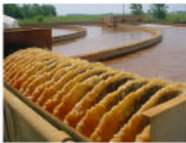
Oxidation ditch at a Cheese plant
